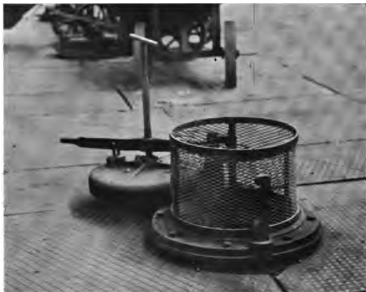
Fig. 4. Guard for Generator Coaling Door.*
